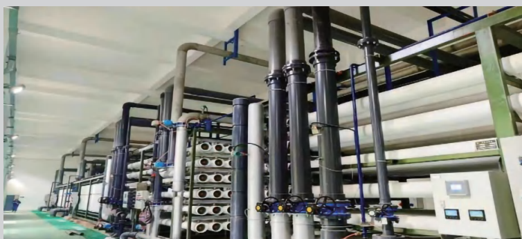
Special waste water treatment system
